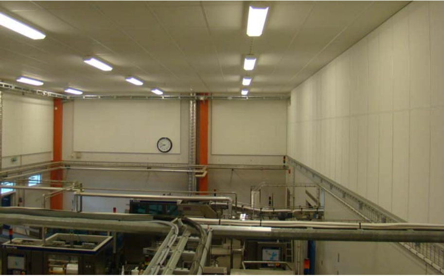
Figure 8. Acoustic treatment of ceiling and walls in Oatly's factory.
