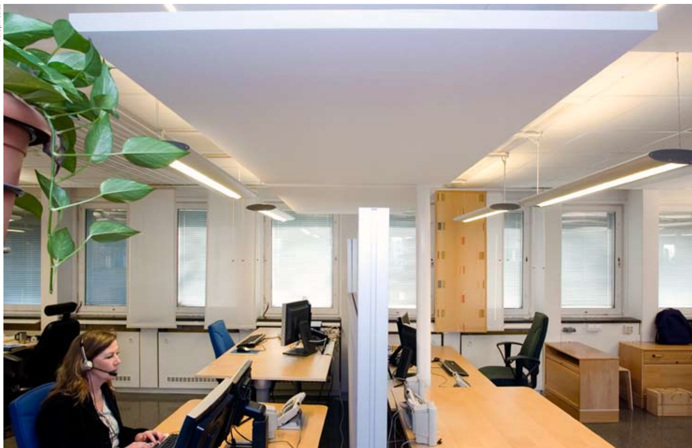
Suspended sound-absorbing units reduce distractions from surroundings and lower sound pressure level.
