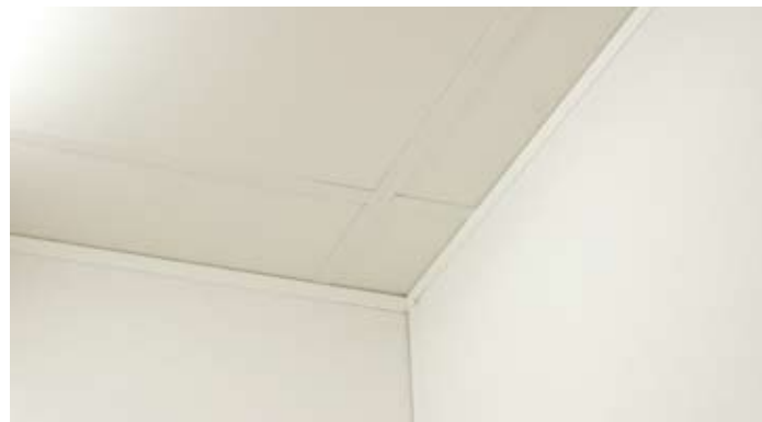
Sound-absorbing materials on the ceilings and walls reduce problems with flutter echoes, for example.
