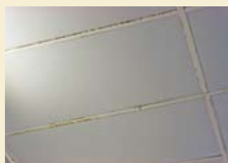
An acoustic ceiling with corroded grid. A grid system of homogenous acid-resistant steel would have been unaffected.
