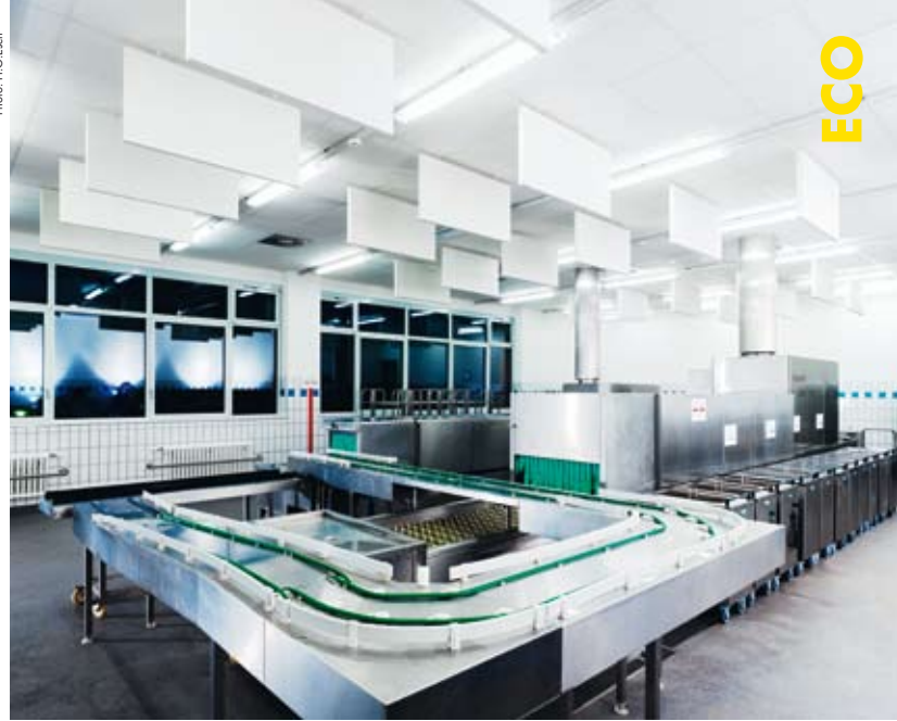
Continuous sound-absorbing panels on the ceiling are combined here with vertical sound-absorbing baffles. Dishwashing areas can otherwise be extremely noisy environments.
