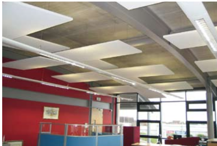
A total of 26 free-hanging sound absorber panels were installed, reducing the reverberation time from 1.68 to 0.7 seconds.
