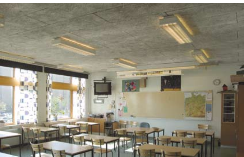
Before. Direct fluorescent light fittings in a wood wool ceiling that has limited sound absorption and does not reflect light effectively around the premises.
